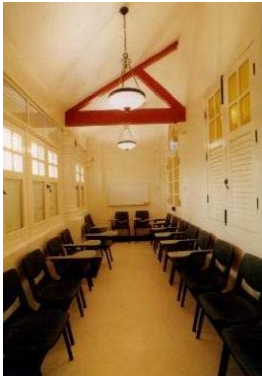
Detail of exposed truss and antique pendant light at Second Floor Balcony
